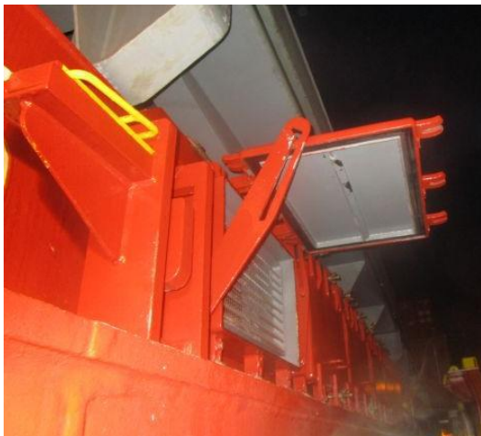
Ref: A typical hatch cover vent flap Transport Malta - Safety Investigation Report – 05/2016
