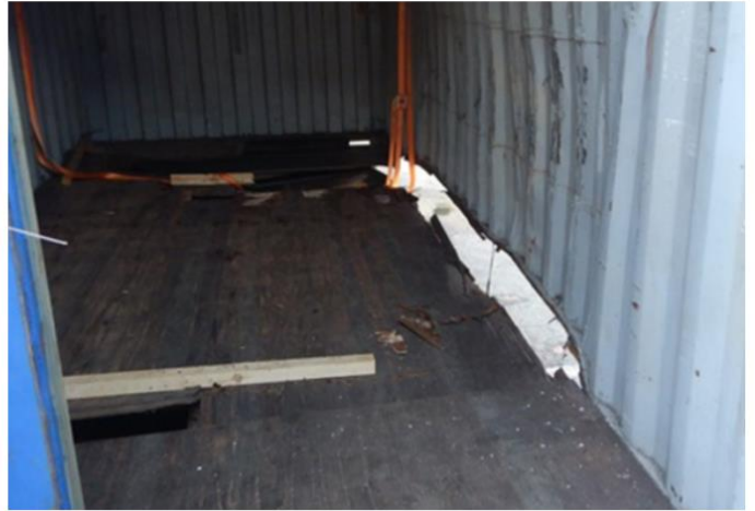
Image: Collapsed Container Floor (Source: Safety Alert 01/2025)
