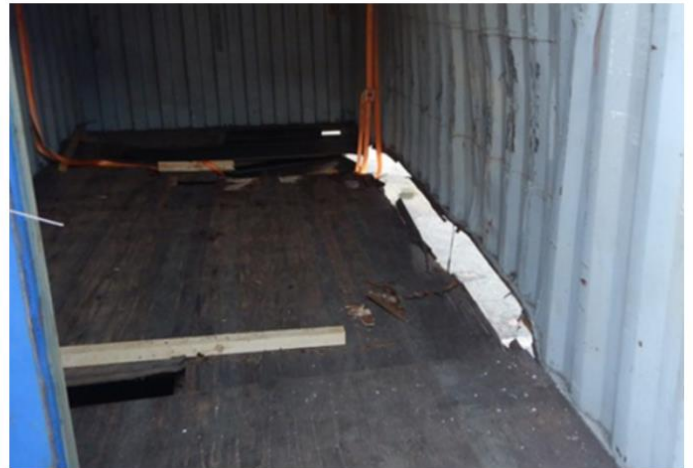
Image: Collapsed Container Floor (Source: Safety Alert 01/2025)
