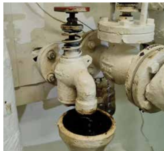
FOST-1 drain valve
