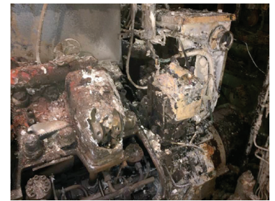
Some of the damage incurred
