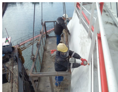
Working at height without a safety harness
