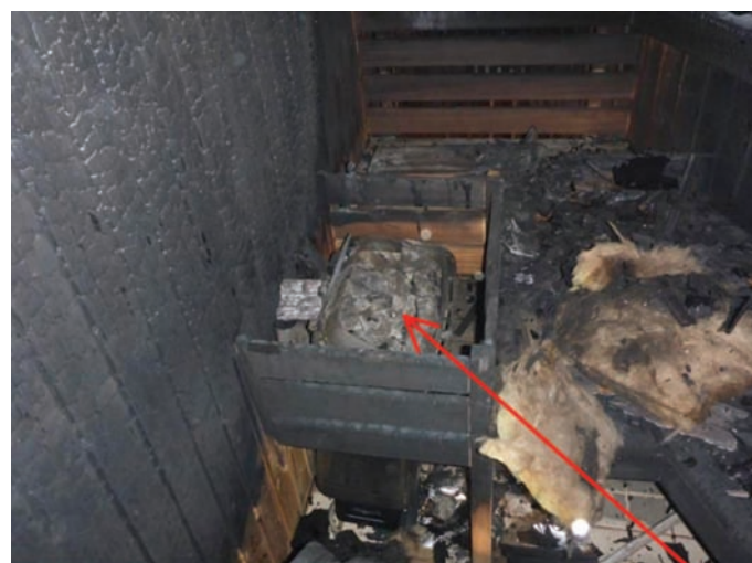
Burned sauna and heater
