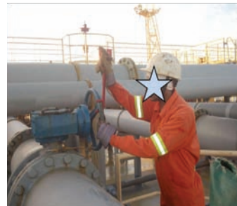
Opening the valve
