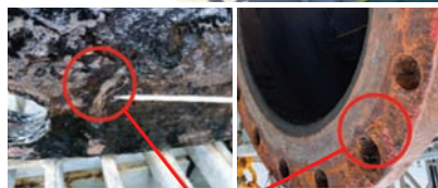
Small groove allowed oil leak
