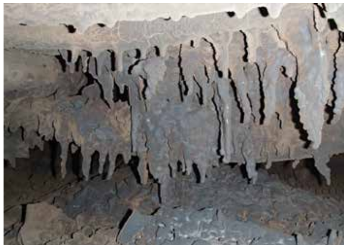
Fire damage to EGE
