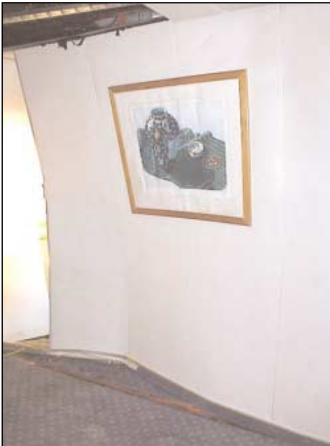
Photograph of distorted bulkhead
