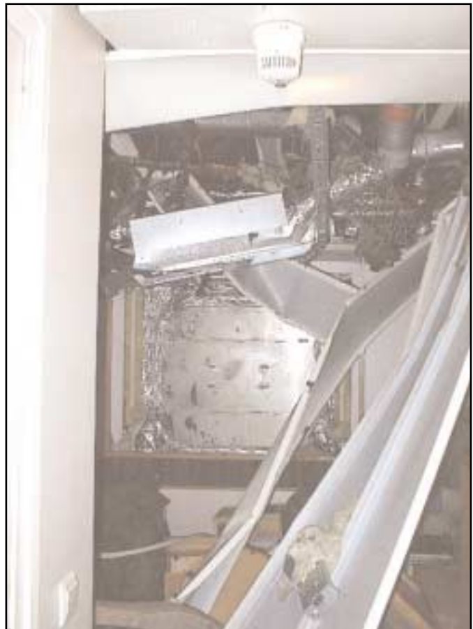
Photograph of damaged ceiling
