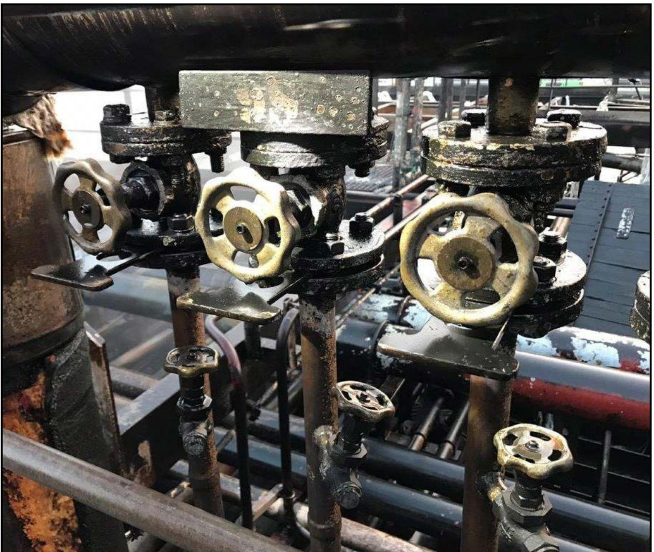
Figure 10: 9S heating control valves
