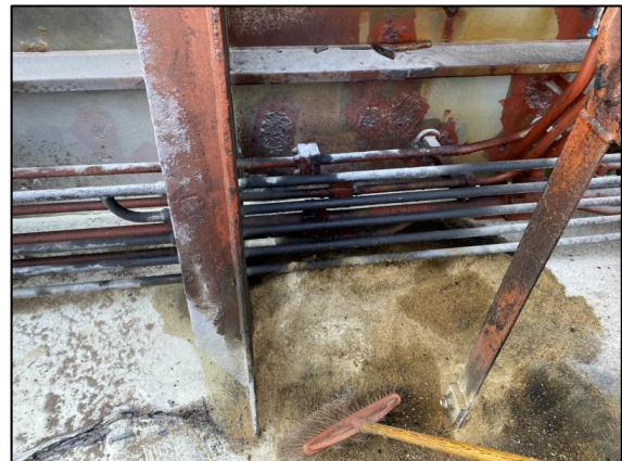
Figure 5: Sawdust soaked with the hydraulic oil that leaked out
