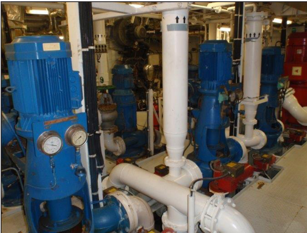
Figure 1: Bilge and ballast pumps and valves
