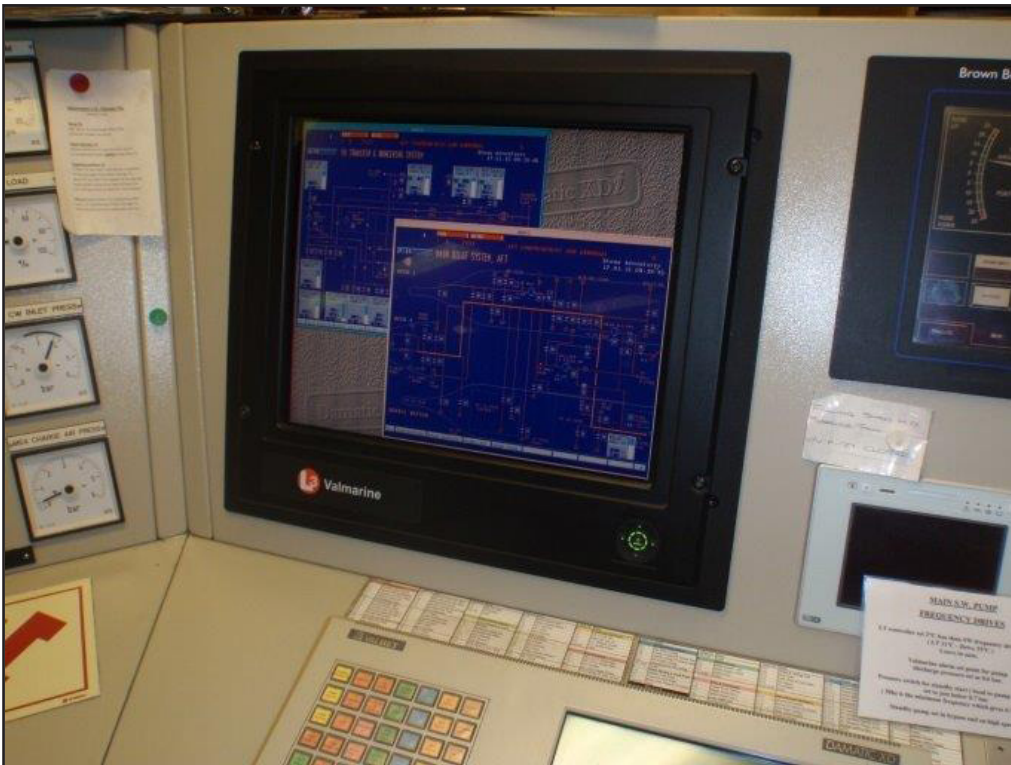
Figure 2: PMS control station
