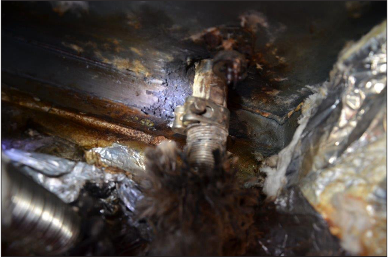
Figure 2: Uninsulated exhaust pipe causing the wooden deck to char
