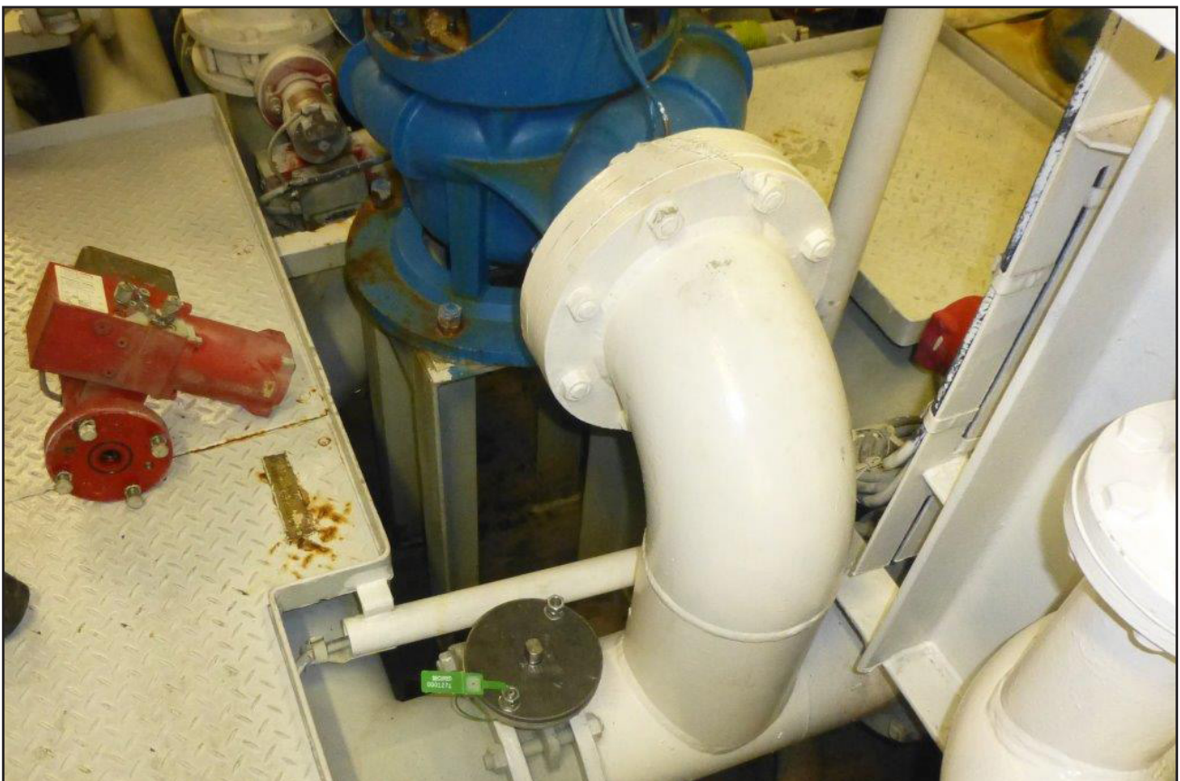
Figure 4: Modified cross-over valve - actuator removed, locking device fitted
