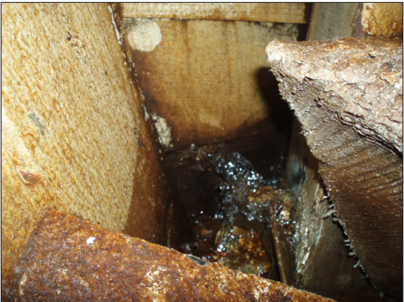
Water ingress between the planks
