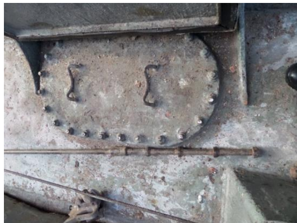
Poor condition of tank cover
