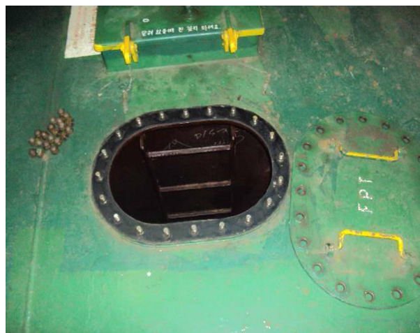
Top side manhole cover
