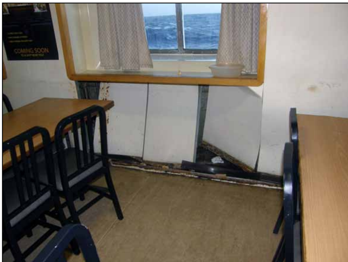
Damage to crew mess room, Deck 3
