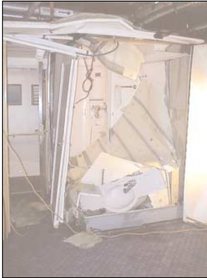
Photograph of damaged bathroom module
