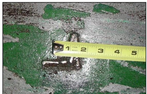
Figure 10: The base of one of the failed welded angle bars
