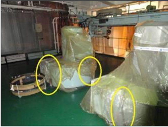
Figure 6: Lashed spare auxiliary blowers in the engine-room
