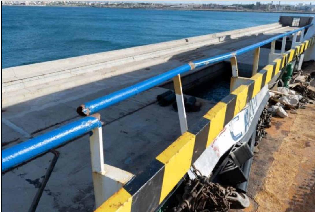
Figure 23: Damaged guard rails
